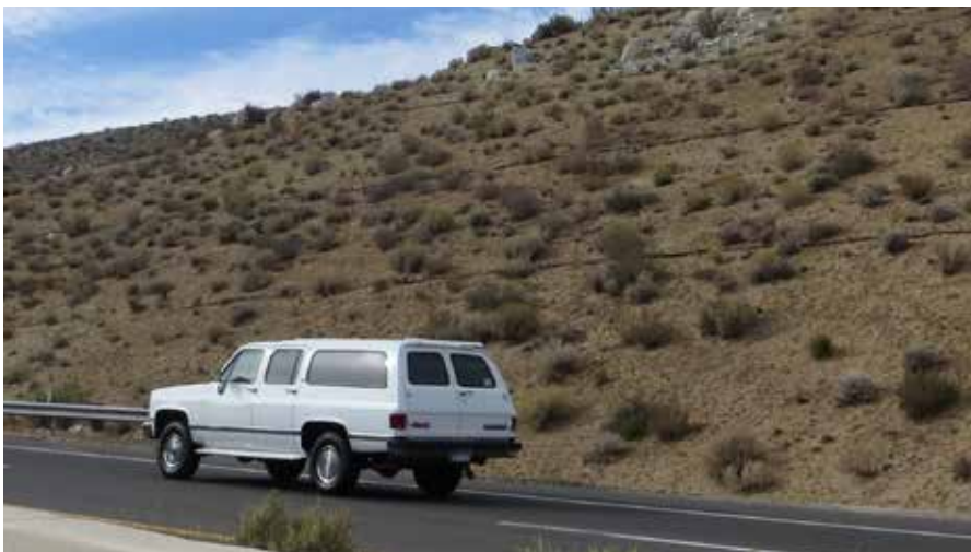
Naturalized rock cuts and grading that blend with the surrounding topography are preferred. Mass grading of slopes is visually unappealing and leads to vegetation management issues.
